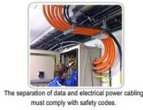
The separation of data and electrical power cabling must comply with safety codes.
